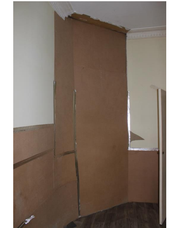
Figure 40: MDF board installed to cover the location of the former fire place in the western front room.
