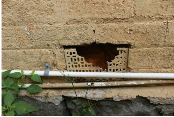
Figure 30: Subfloor vent which has been filled with expanding foam
