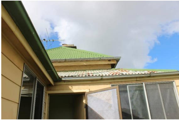
Figure 23: View south to entry to rear addition clad in Hardi plank boards.
