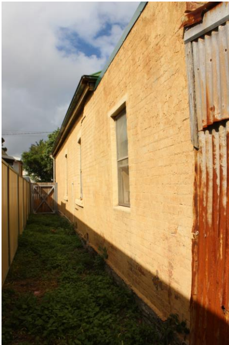
Figure 31: East elevation showing the junction of the original brick wall with the corrugated galvanised walls of the laundry addition.
