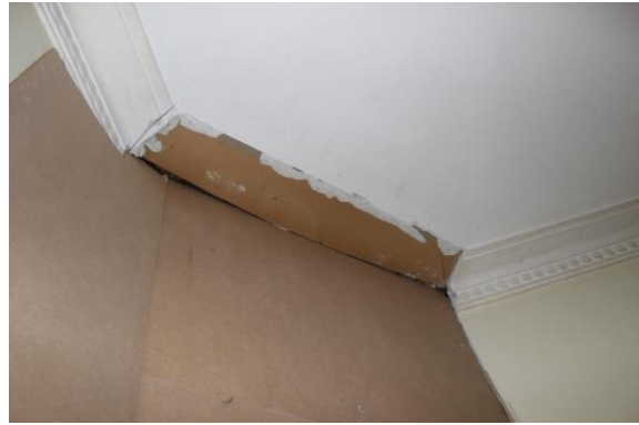
Figure 36: MDF board installed to cover the location of the former fire place in the western front room.
