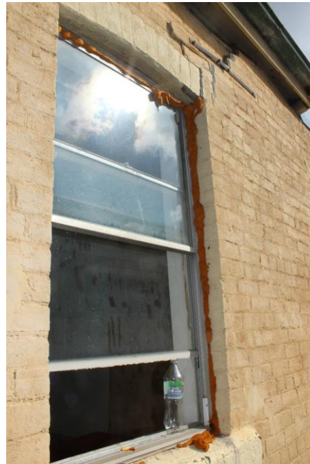
Figure 32: Original window opening on the east elevation. The original timber windows have been removed and replaced with ill-fitting aluminium windows and the gaps filled with expanding foam
